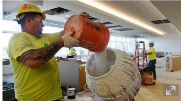
Rodolfo Exposito mixes terroxy material for pouring onto the third floor elevator lobby leading into the check-in and check-out patient area. (Taimy Alvarez / Sun Sentinel)
