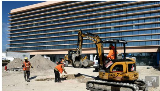
Construction crews work outside the front entrance to the new Cleveland Clinic Florida's neurological and cancer center. (Taimy Alvarez / Sun Sentinel)
