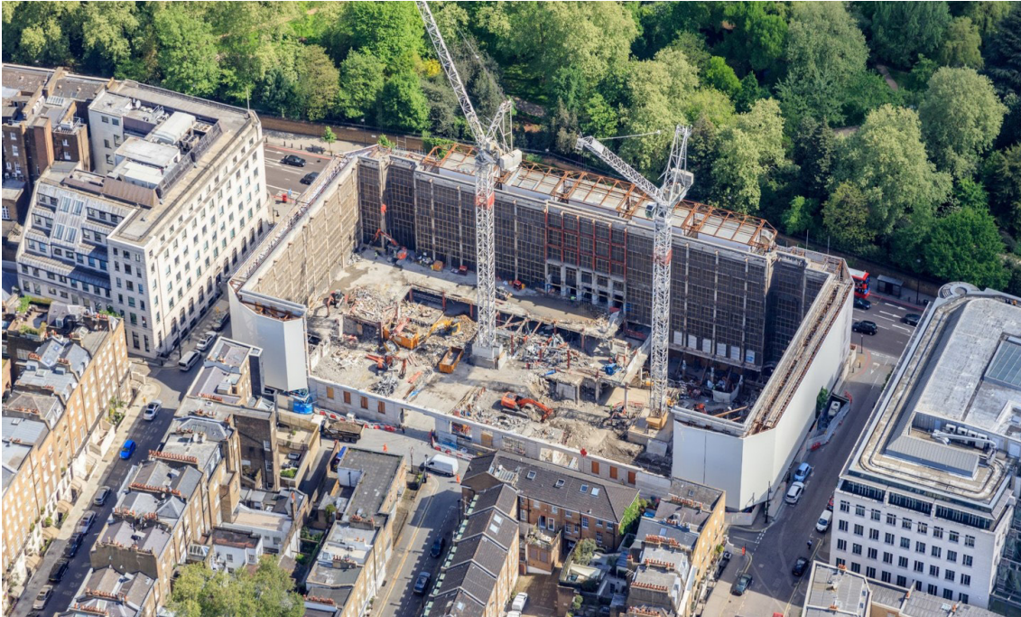
May 2018. The building that will become Cleveland Clinic London is gutted, preparing for the new hospital.
